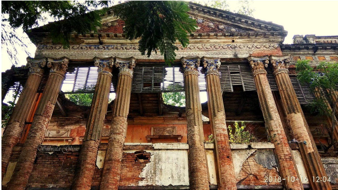
Image No 97: The Dilapidated Mansion Of Nimita Rajbari, Subrata Ghose, PKG
